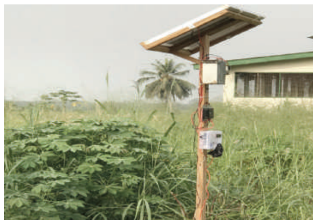
The main drip irrigation control system. It is made up of the solar panel, the battery, the embedded microcontroller system and the submerged bucket, serving as water reservoir.
